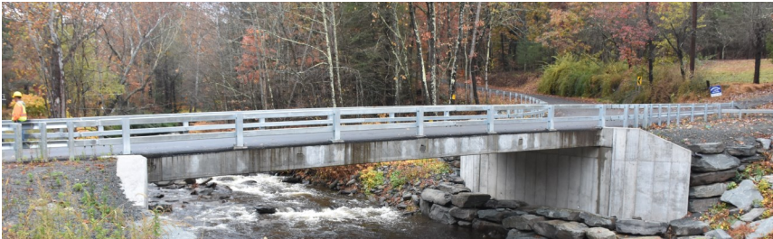
Sandburg Creek rushes below the new Tempaloni Road bridge near Spring Glen in the Town of Mamakating. The $730,000 project included more than just the bridge's concrete beams but also the abutments, guardrails and approaches on either side.
