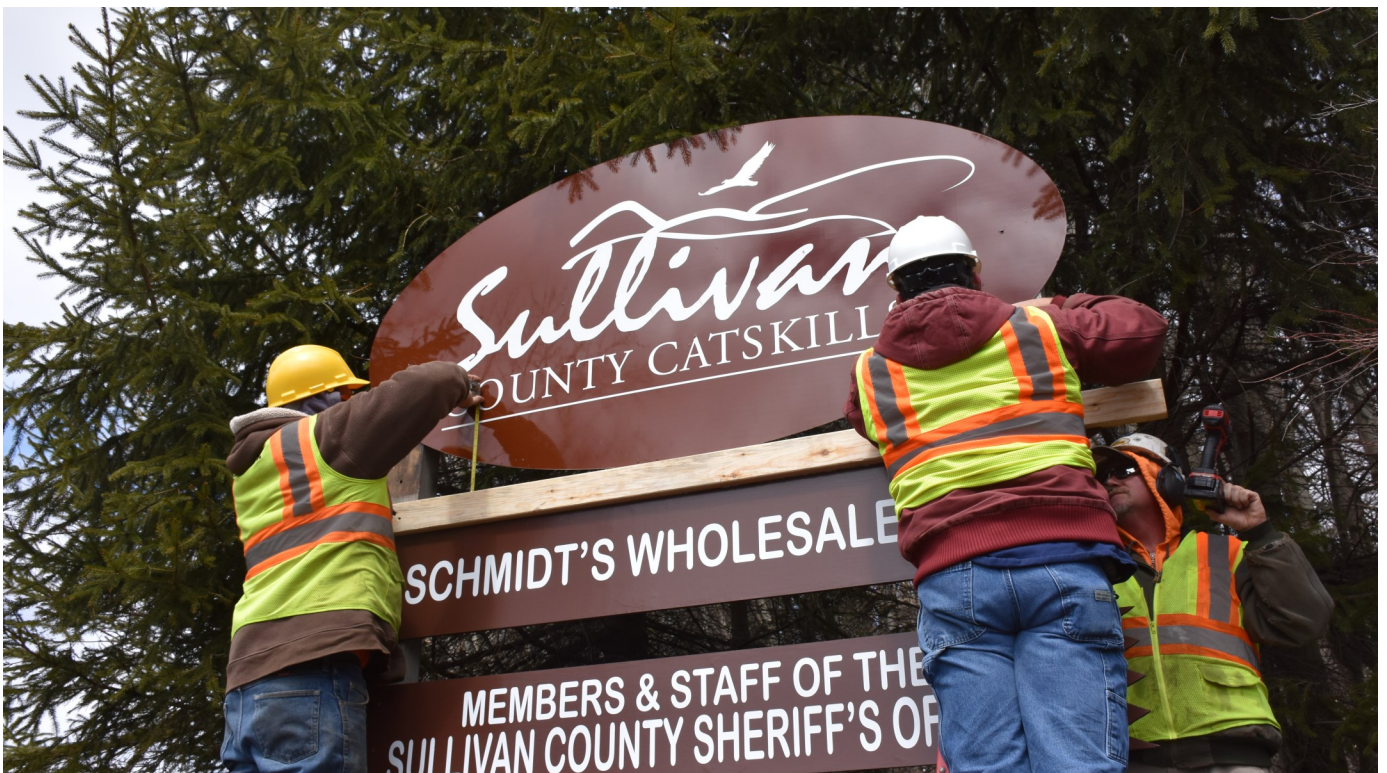
They may be camera-shy, but they're mighty efficient! Caught putting up the new Adopt-an-Exit signs along Route 17 last month were installers Pat Kerr and Pete Finck, plus Sign Shop Supervisor Charlie Kocher. And yes, the signs were made in our own Shop!
